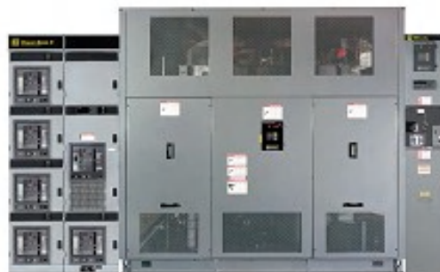
Figure 3 Distribution Transformer with Built-in Webserver
